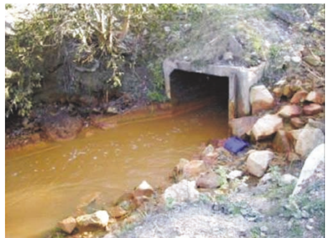
Mine Drainage Water
